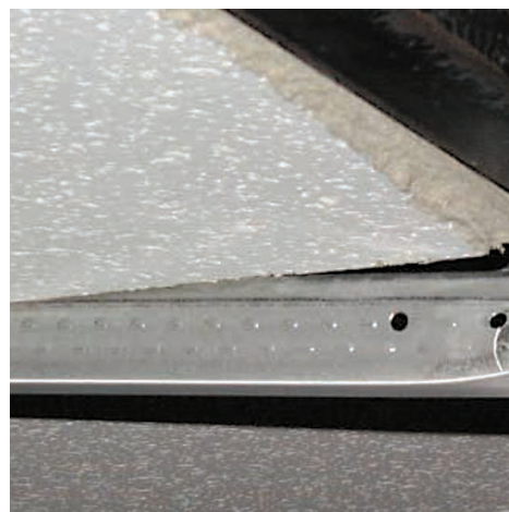
Unsupported cross tees allow panels to drop out.
