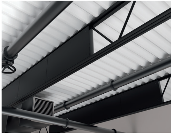
InvisAcoustics™ Panels in Black Truss Installation
