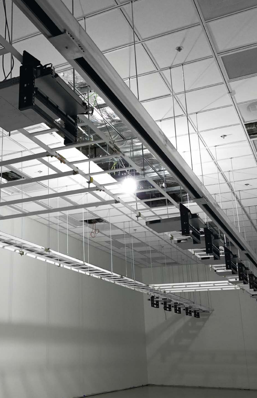
DynaMax® Structural Grid Data Center Installation
