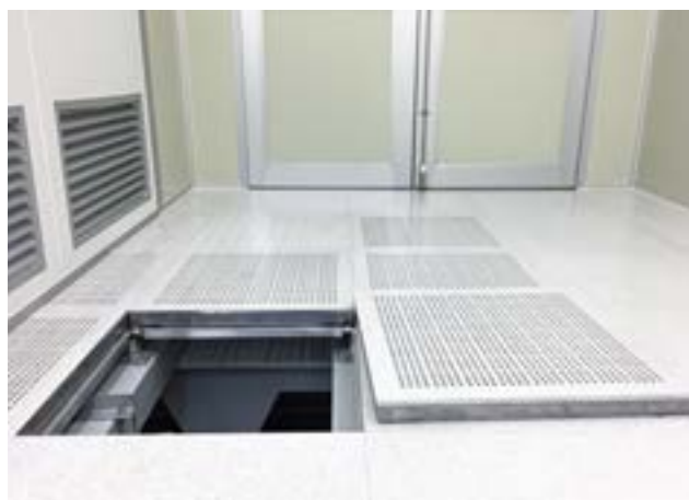
Raised Floor Data Center
