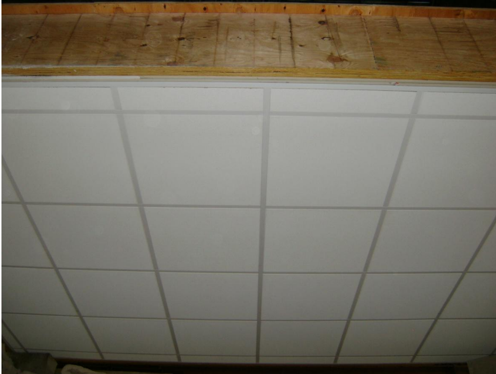
Figure 6. Exposed surface of comparative floor/ceiling assembly protected with AWI suspended ceiling tile system
