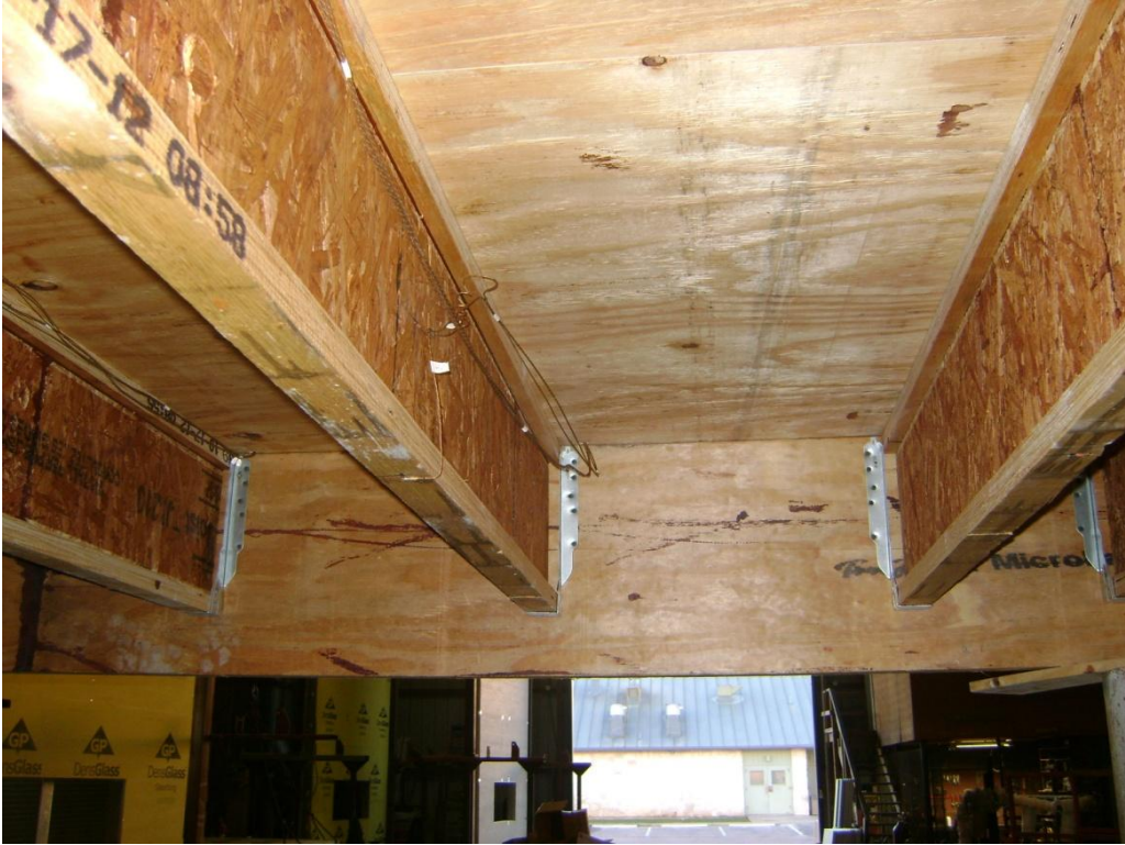
Figure 4. Underside of floor/ceiling assembly prior to installation of membrane protection system (typical)
